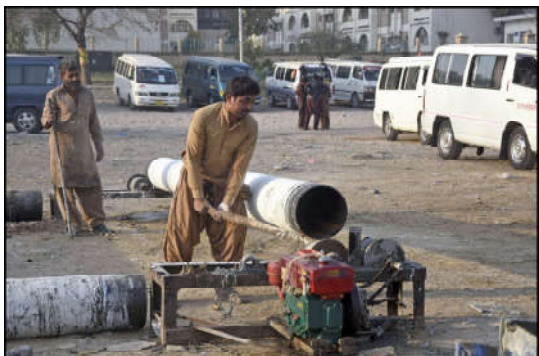
ISLAMABAD: Labourers are busy installing new water pipeline at sector F-5 in the Federal Capital.
