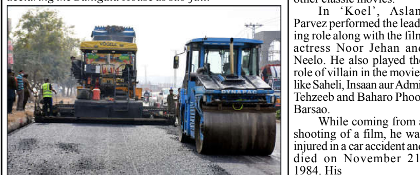
ISLAMABAD: Labourers are busy in carpeting at a road in the Federal Capital.
