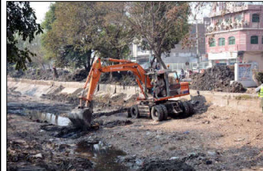
FAISALABAD: Irrigation department worker clearing a Rakh Branch canal with the help of caterpillar during canal cleaning campaign
