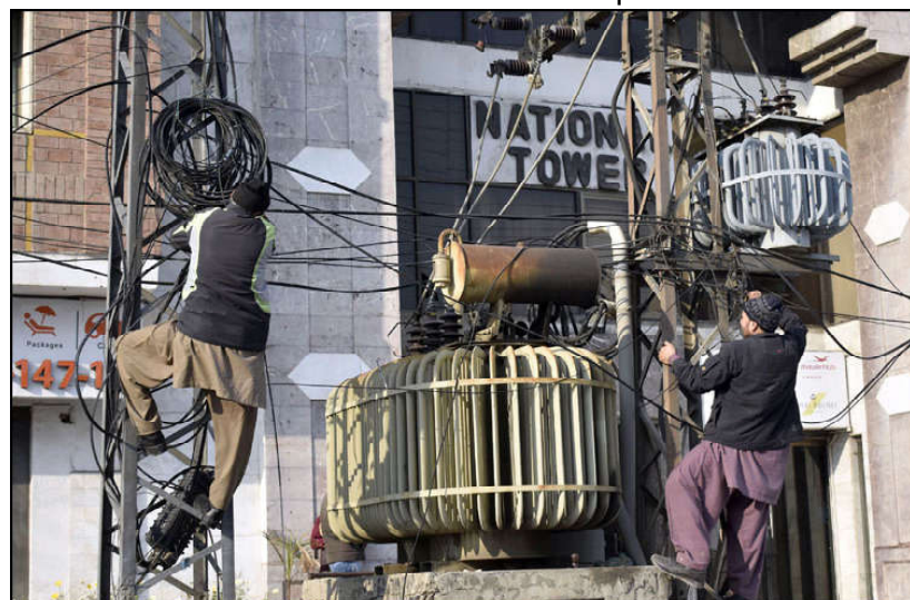
LAHORE: Workers of WAPDA are busy in repairing Transformers on electric poles alongside a road, in Provincial Capital.
