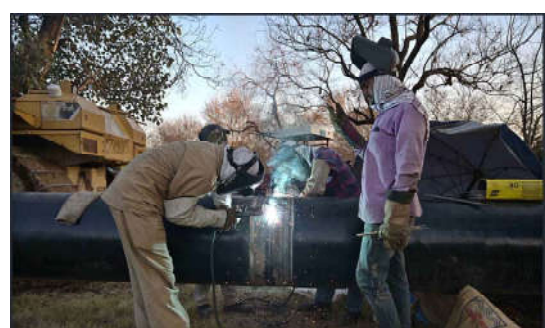
ISLAMABAD: Workers welding pipes of gas line at Aabpara area in the federal capital.
