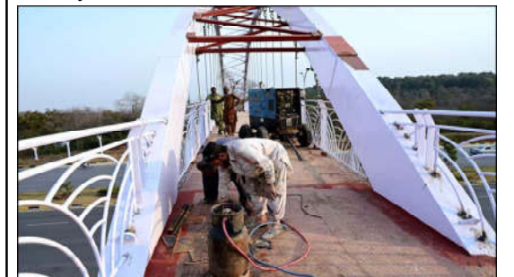
ISLAMABAD: A welder finishing grills of a new pedestrian bridge over the Srinagar Highway in the Federal Capital.
