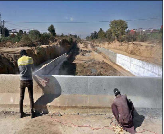
ISLAMABAD: Labourers busy in construction work of bridge on under construction 10th Avenue during development work in Federal Capital.
