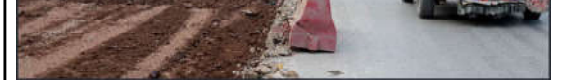
ISLAMABAD: Labourers busy in construction work of Park Road with the help of heavy machineries during development work in the city.
