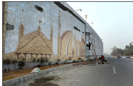
ISLAMABAD: Laborers busy in construction work to enhance the beauty of the city on the wall of a flyover at Rawal Dam Chowk in the Federal Capital.
