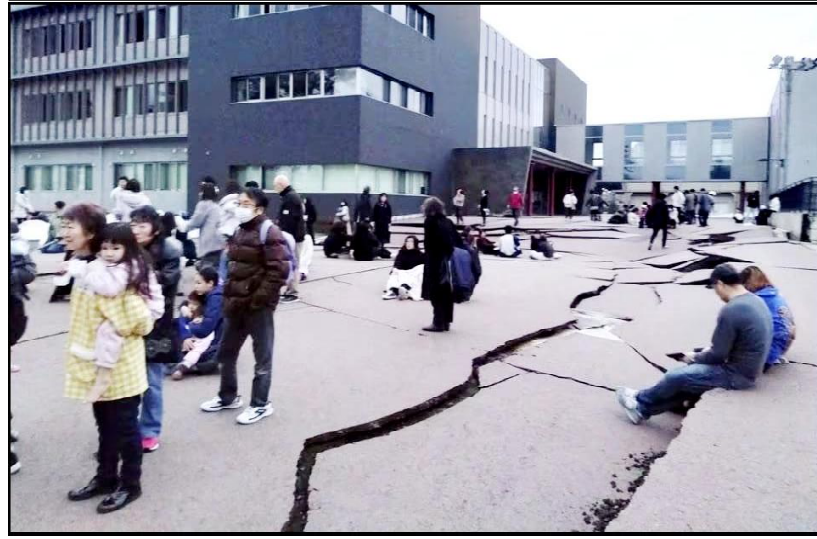
Road cracks caused by an earthquake is seen in Wajima, Ishikawa prefecture, Japan
