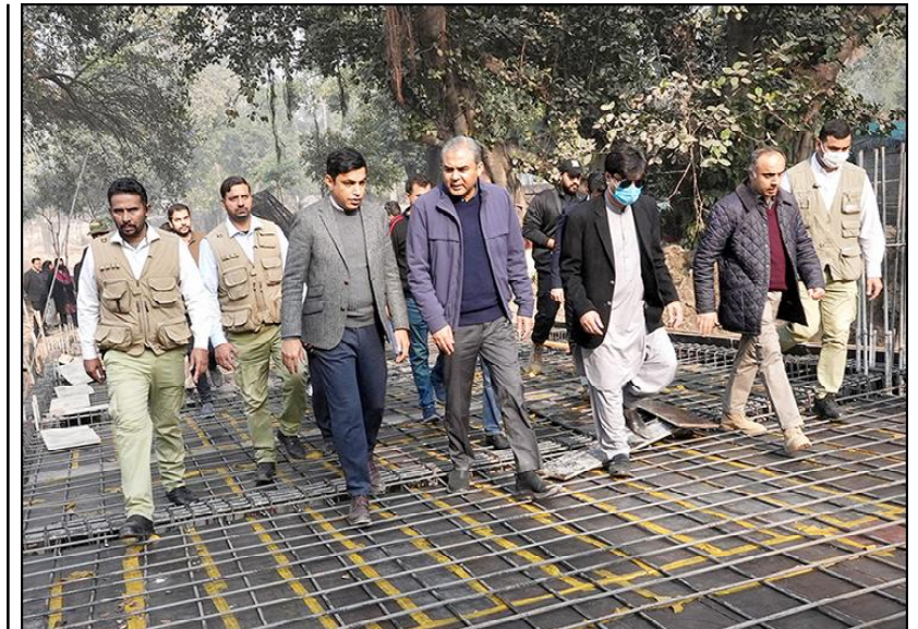
LAHORE: Caretaker Chief Minister Punjab Mohsin Naqvi inspecting the on-going construction works at Lahore Zoo.
