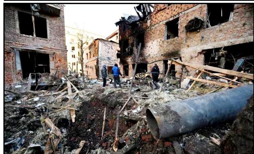
Residents inspecting the damage outside an apartment building after the overnight Russian drone attack in Kharkiv.
