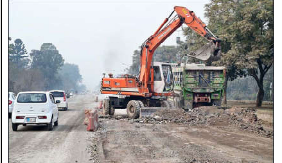
ISLAMABAD: Machinery being used for extension work of Park Road during development work in the Federal Capital.
