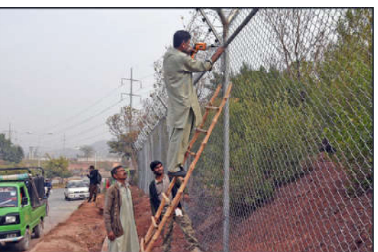
ISLAMABAD: Workers are busy in installing electric fence around diplomatic enclave in Federal Capital.
