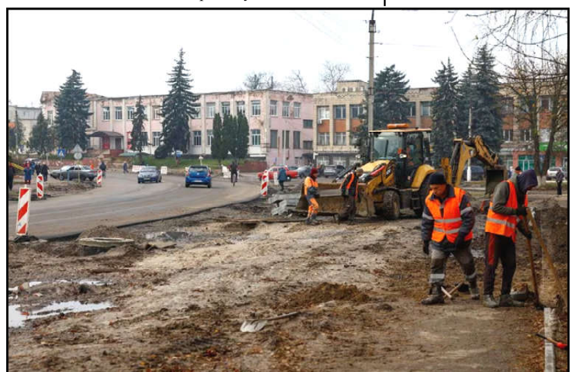
Workers reconstruct a street, which was damaged on the first months of Russia's attack on Ukraine in the town of Trostianets, Sumy region, Ukraine.
