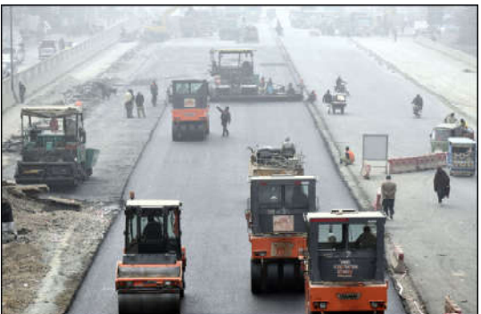
LAHORE: Labourers are busy in construction work of Sagian Road with the help of heavy machinery in the Provincial Capital.
