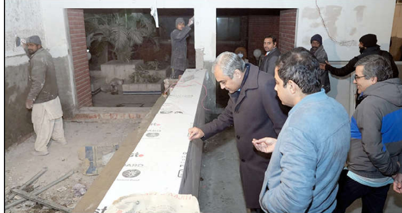
LAHORE: Caretaker Chief Minister Punjab Mohsin Naqvi inspecting the construction work of the reception counter under upgradation project during his visit to Children Hospital.
