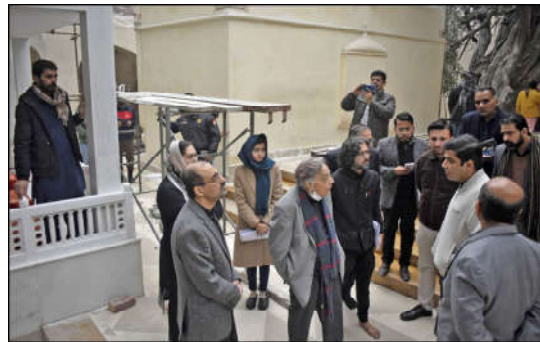
LAHORE: Deputy Commissioner Rafia Haider along with Secretary Aqaf Dr. Syed Tahir Raza Bukhari being briefed during their visits to the site of under construction Shrine of Bibi Pak Daman, in Provincial Capital.
