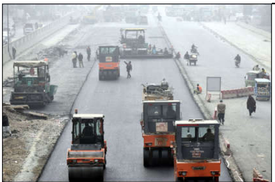
LAHORE: Labourers are busy in construction work of Sagian Road with the help of heavy machinery in the Provincial Capital.
