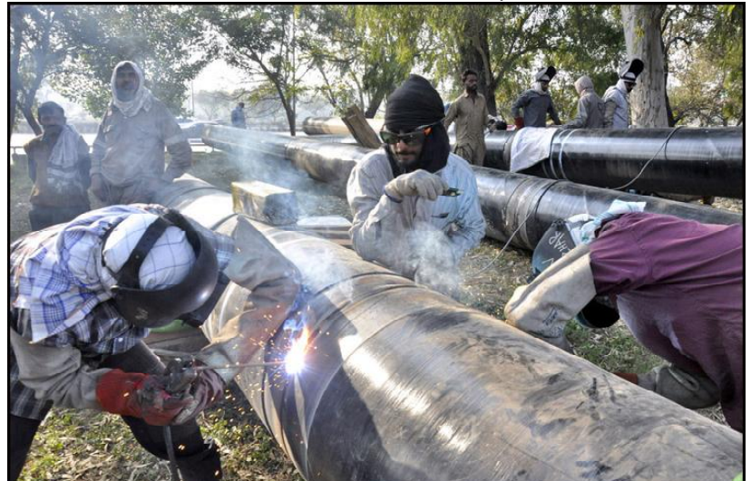
ISLAMABAD: SNGPL staffs welding gas pipes installing at Zeropoint area in federal capital.
