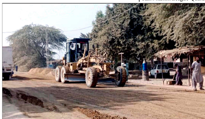
HUB: Heavy machineries busy in construction work of road carpeting of the one-way road under the supervision of local government departments, located on Sakran area in Hub
