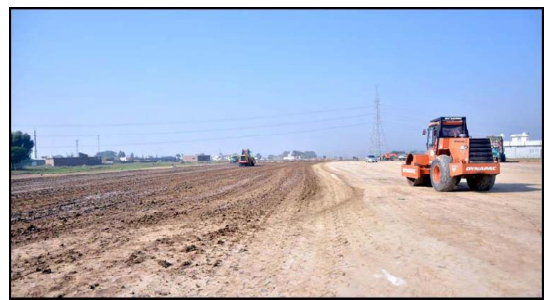
ISLAMABAD: Heavy machinery being used to build Chak Beli Link Road in the outskirts of the city.
