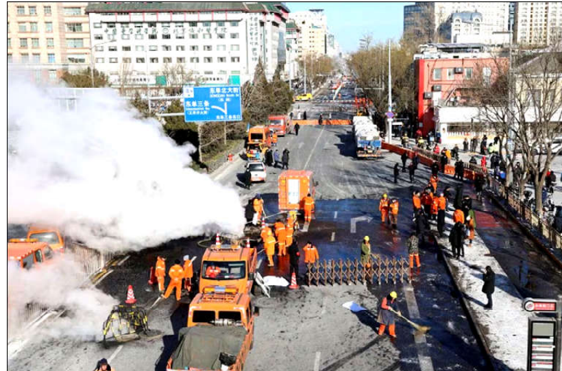
Workers conduct repair work at the site where a thermal pipeline that supplies heating leaked, during winter solstice in Beijing, China.
