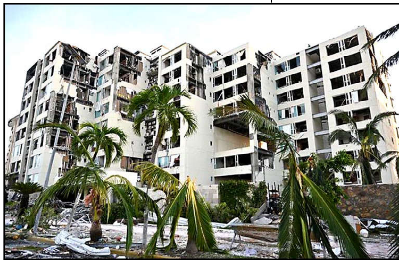
MEXICO: A view of damaged buildings due to Hurricane Otis made landfall near Acapulco.
