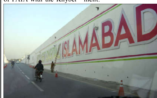
ISLAMABAD: Laborers are busy in decorate paint wall of Rawal Dam underpass "Let's Get Digital Islamabad" in the Federal Capital.
