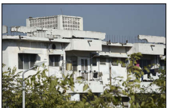
ISLAMABAD: A view of weary condition residential building at sector G-11 in Federal Capital, which may cause any incident any time as needs to attention for concern authority.
