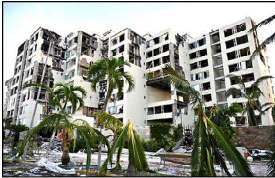
MEXICO: A view of damaged buildings due to Hurricane Otis made landfall near Acapulco.
