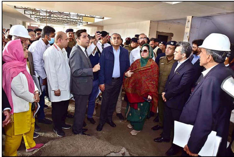
FAISALABAD: Chief Minister Punjab, Syed Mohsin Raza Naqvi is visiting the Allied Hospital Faisalabad to inspect ongoing upgradation projects of Surgical Emergency and OPD Wards.
