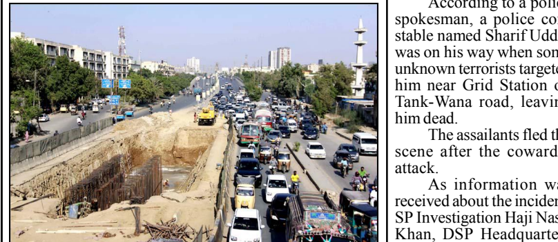
KARACHI: Construction works of new development projects is underway under the supervision of local government department, as slow pace of construction work is creating problems for commuters due to traffic jam and they demand to concerned department to complete work as soon as possible, located near Nipa Chowranghi at University road in Karachi.
