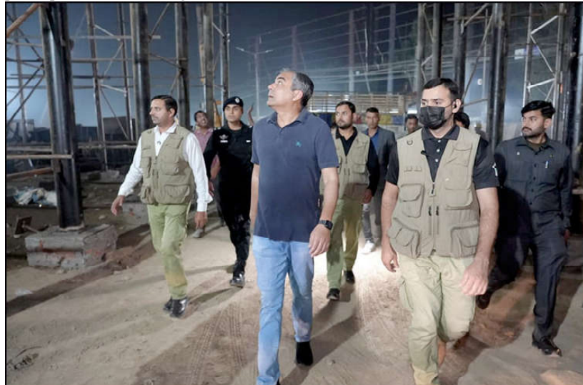
LAHORE: Caretaker Chief Minister Punjab Mohsin Naqvi inspecting the steel fixing works of Ghora Chowk Defence Morr Flyover Project.
