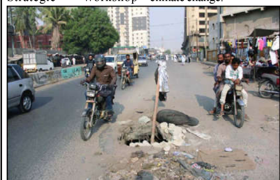
KARACHI: Commuters pass through nearby an open sewerage main hole that may cause any accident specially in night hours, showing the negligence of concerned departments, at Saddar area near Parking Plaza in Karachi.
