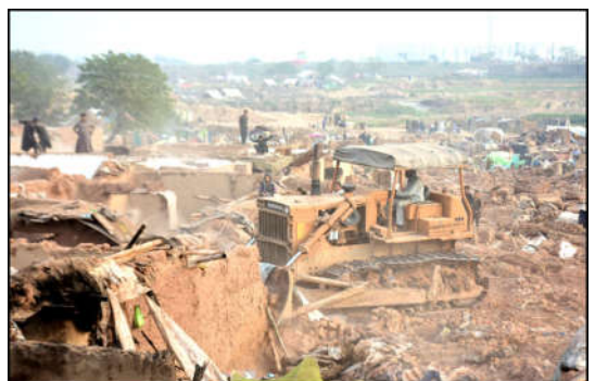
ISLAMABAD: Workers are demolishing the illegally contracted houses at Afghan Basti I-12 as Pakistani Authorities announce warning for people living in Pakistan illegally to leave the country as Pakistani security forces on Wednesday rounded up, detained and deported dozens of Afghans who were living in the country illegally, after a government-set deadline for them to leave.
