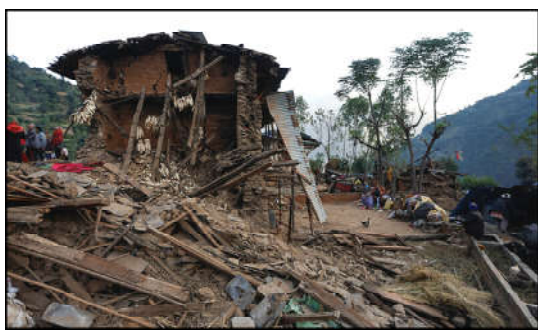
Debris of houses collapsed during an earthquake are pictured in Jajarkot, Nepal.
