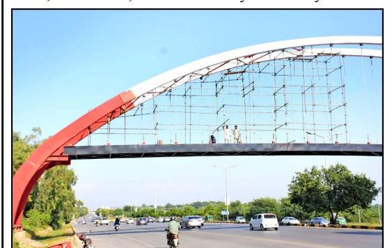
ISLAMABAD: Workers are busy in giving final touch to the newly installed over head pedestrian bridge at Srinagar Highway in Federal Capital.
