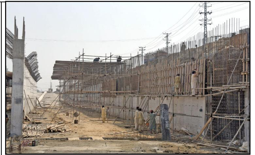
ISLAMABAD: Laborers are busy in their work during the construction of Golra Mor Underpass in Federal Capital.
