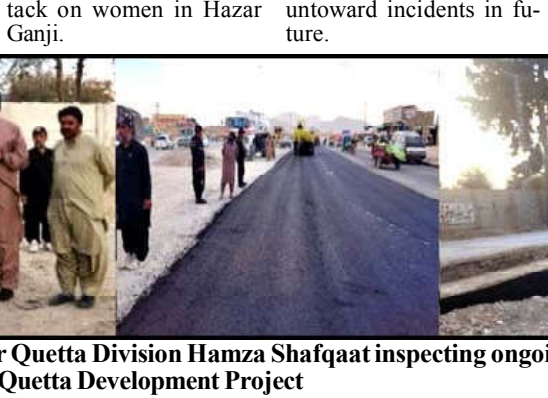
QUETTA: Commissioner Quetta Division Hamza Shafiqat inspecting ongoing works of Sariab Road and other projects under Quetta Development Project
