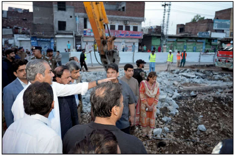
LAHORE: Caretaker Chief Minister Punjab Mohsin Naqvi issuing directives regarding construction works during his visit to under construction controlled access corridor project.
