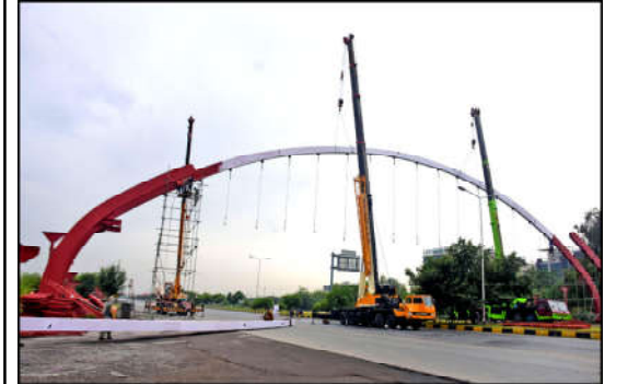
ISLAMABAD: Workers of local administration are busy in installing over head pedestrian bridge with the help of heavy machinery at Srinagar Highway as the main busy highway will be closed for two days in Federal Capital.
