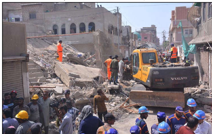
KARACHI: Rescue workers searching at site where an under-construction building collapsed. 5 dead, 4 injured as under-construction building collapses in Karachi's Shah Faisal Colony.
