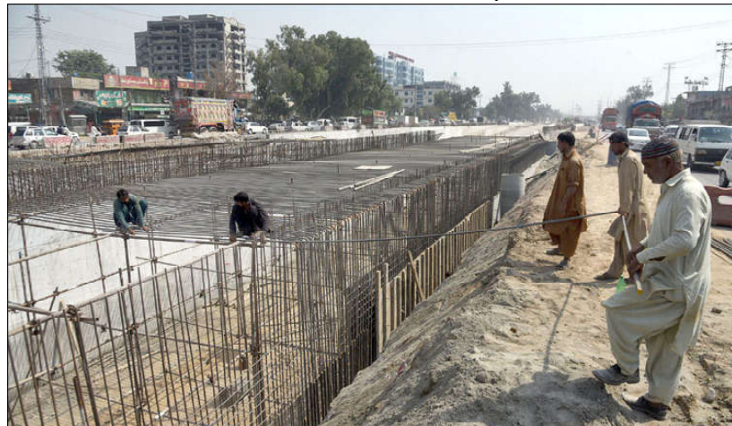
ISLAMABAD: Laborers are busy in their work during the construction of Golra Mor Underpass in Federal Capital.
