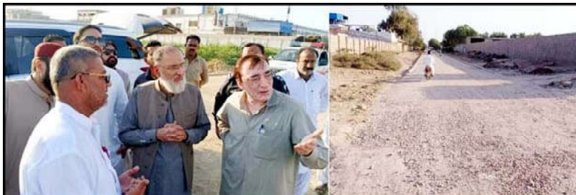
HUB: Caretaker Provincial Minister for Industries, Excise and Taxation Prince Ahmed Ali Ahmedzai issuing directives to MLIEDA during his visit to site of under construction road network project
