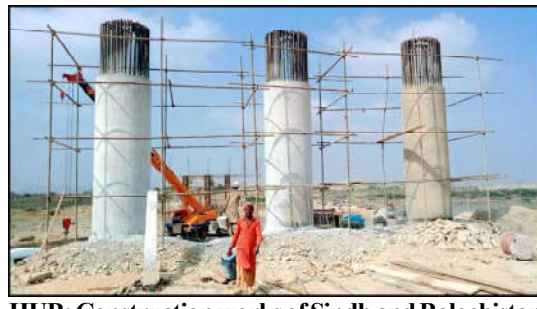
HUB: Construction works of Sindh and Balochistan connecting Bridge is underway, in Hub.
