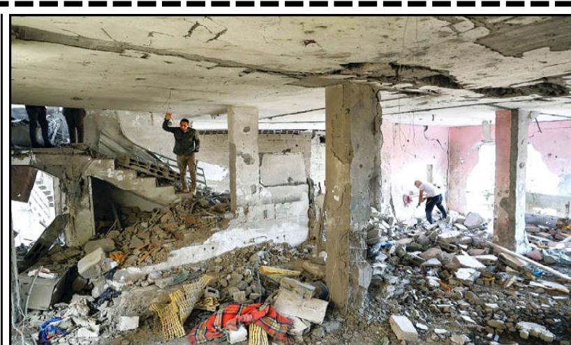
Palestinians check the damage inside a mosque which was hit in an Israeli air strike, in Jenin refugee camp in the Israeli-occupied West Bank.
