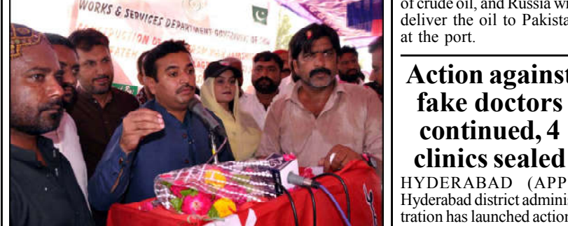
HYDERABAD: Mayor Hyderabad, Kashif Ali Shoro addresses after inaugurating the construction works of road, at Al-Fateh Town located on Qasimabad in Hyderabad.
