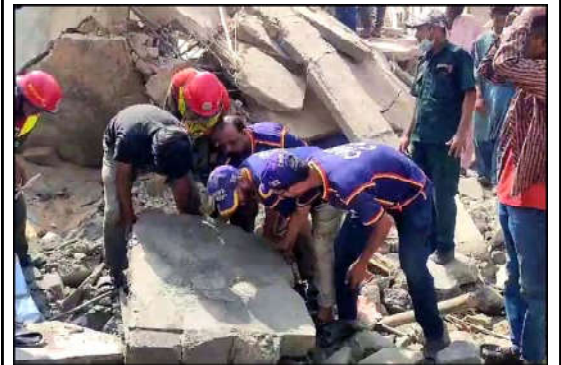
KARACHI: View of site after under-construction building collapse incident as rescue operation is underway, at Shah Faisal Colony area in Karachi.
