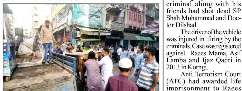
KARACHI: Anti encroachment operation in progress removed illegal encroachment during anti encroachment drive under the supervision of District Municipal Corporation (DMC South), located on Cycle Market Light House in Karachi.
