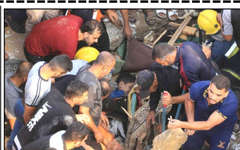
Palestinians recover a body from under the rubble of a building destroyed in an Israeli airstrike in Khan Yunis in the southern of Gaza Strip.
