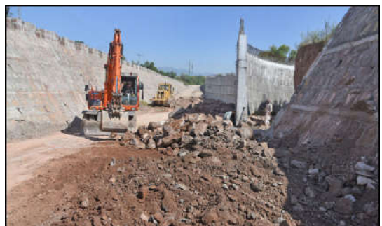
ISLAMABAD: Laborers are busy in their work during the construction of Margala Town Under pass, as the construction work is resume, which was halted due to improvements in the design.
