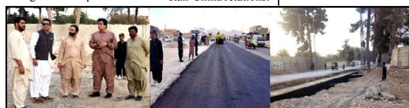
QUETTA: Commissioner Quetta Division Hamza Shafqaat inspecting ongoing works of Sariab Road and other projects under Quetta Development Project
