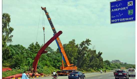
ISLAMABAD: Workers of local administration are busy in installing overhead pedestrian bridge at Srinagar Highway in Federal Capital.
