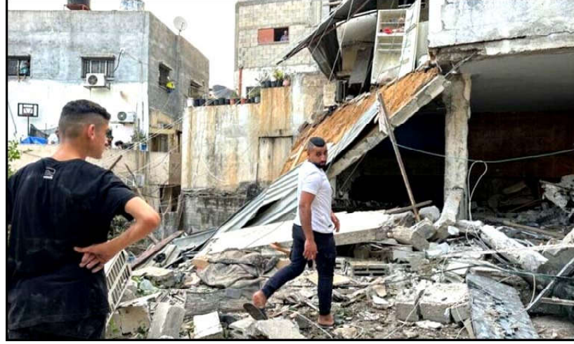
Palestinians check a damaged house following an Israeli raid in Tulkarm in the Israeli-occupied West Bank.
