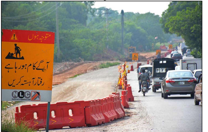
ISLAMABAD: Extension work of Park Road is in process during development work in the Federal Capital.
