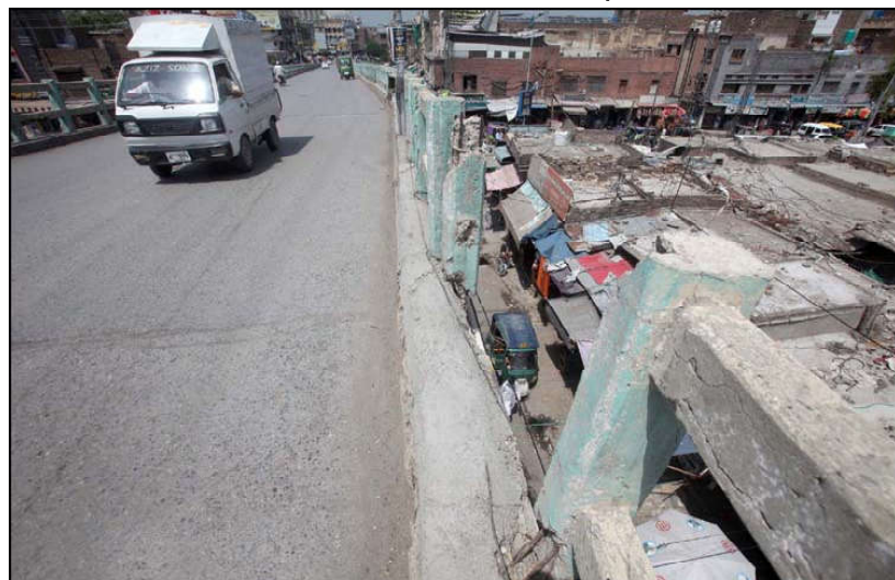
PESHAWAR: Safety wall of Faqirabad Bridge seen broken that may cause any accident and also inviting authorities to draw their attention towards issue, in Peshawar.
