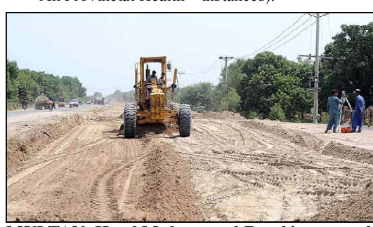
MULTAN: Head Muhammad Road is currently undergoing expansion to ensure smoother traffic flow. This vital route connects several cities in South Punjab, Balochistan, and Khyber Pakhtunkhwa (KPK).
